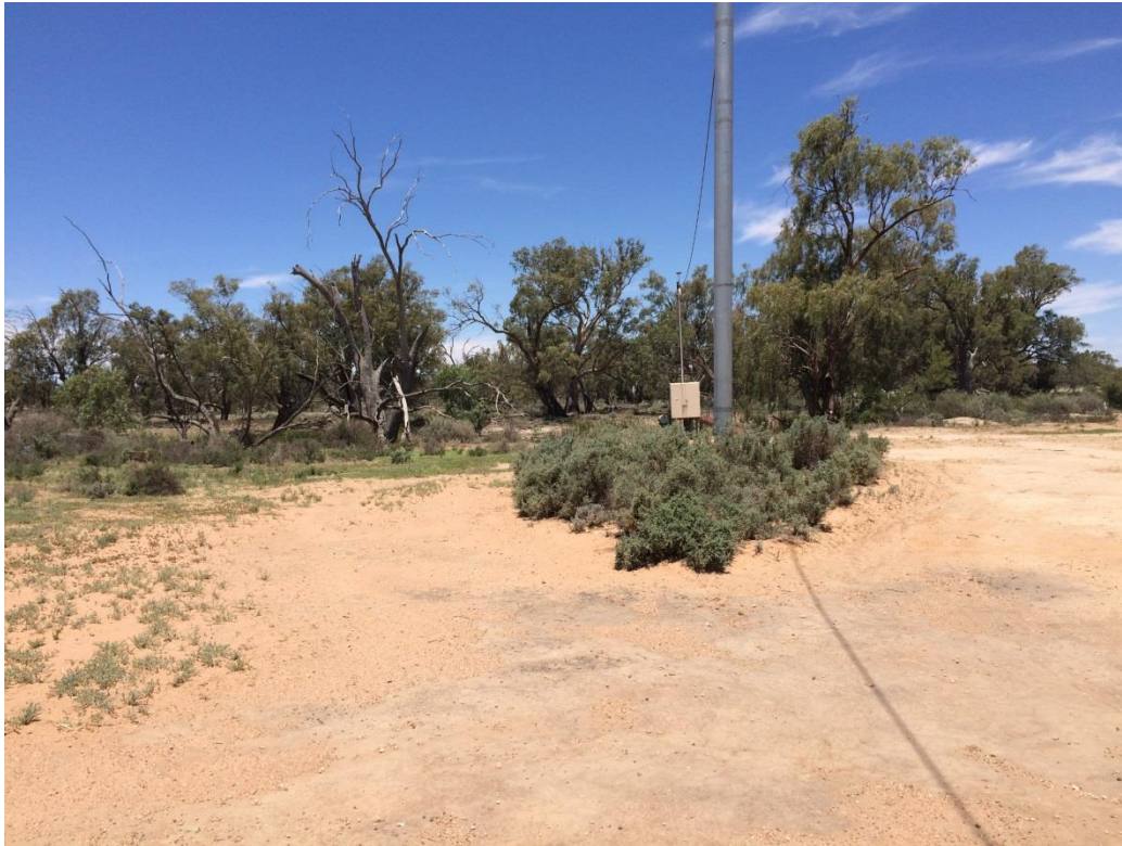
South Pomona – electricity line
